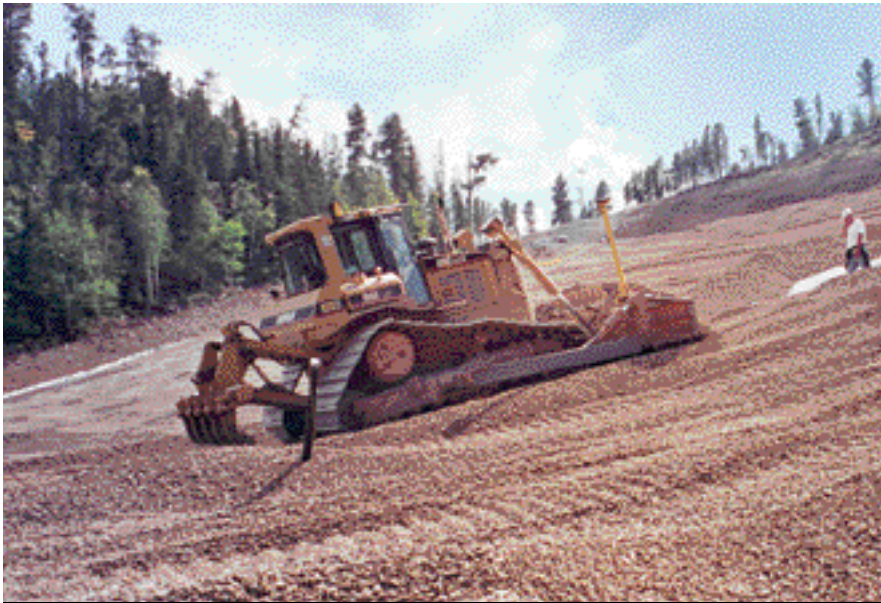
Photo 3. Placement of overlying drain layer using an LGP dozer equipped with GPS for layer thickness control.
