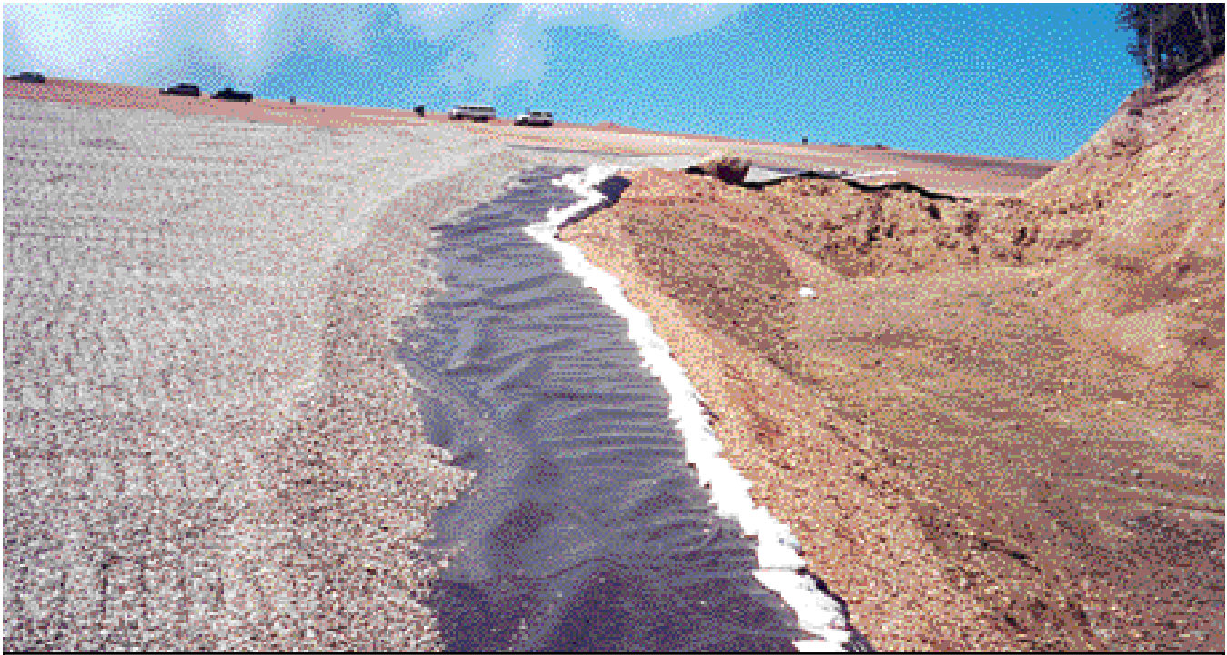
Photo 4. Typical slope area showing open rough cut ditch, ore base, geomembrane system and overlying drain layer—prior to final ditch lining.
