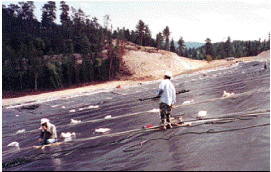
Photo 1. Structured 80-mil LLDPE on slope between benches. Note the smooth surface prior to placement of geotextile and drainage layer.
